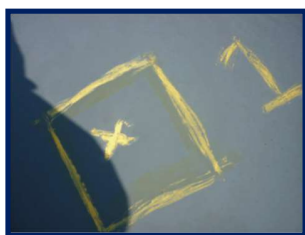
Small breaches found on the roof
