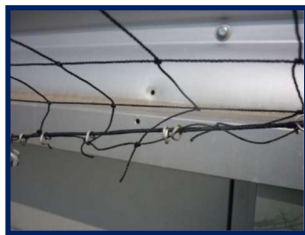
Some of the many missing fixings where leaks occur
